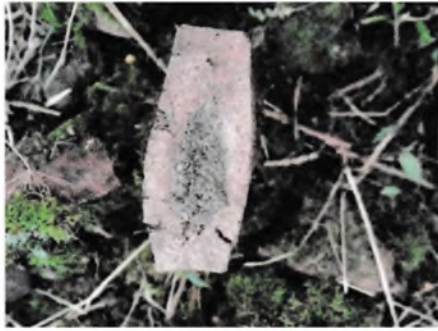
Fig.11 A bloated brick found on the site during a later visit.
