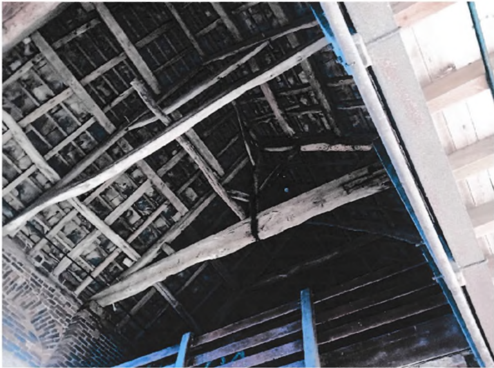
Fig.9 Roof construction of the Great Barn, showing at bottom left the brick arched door opening, later partly filled in.
