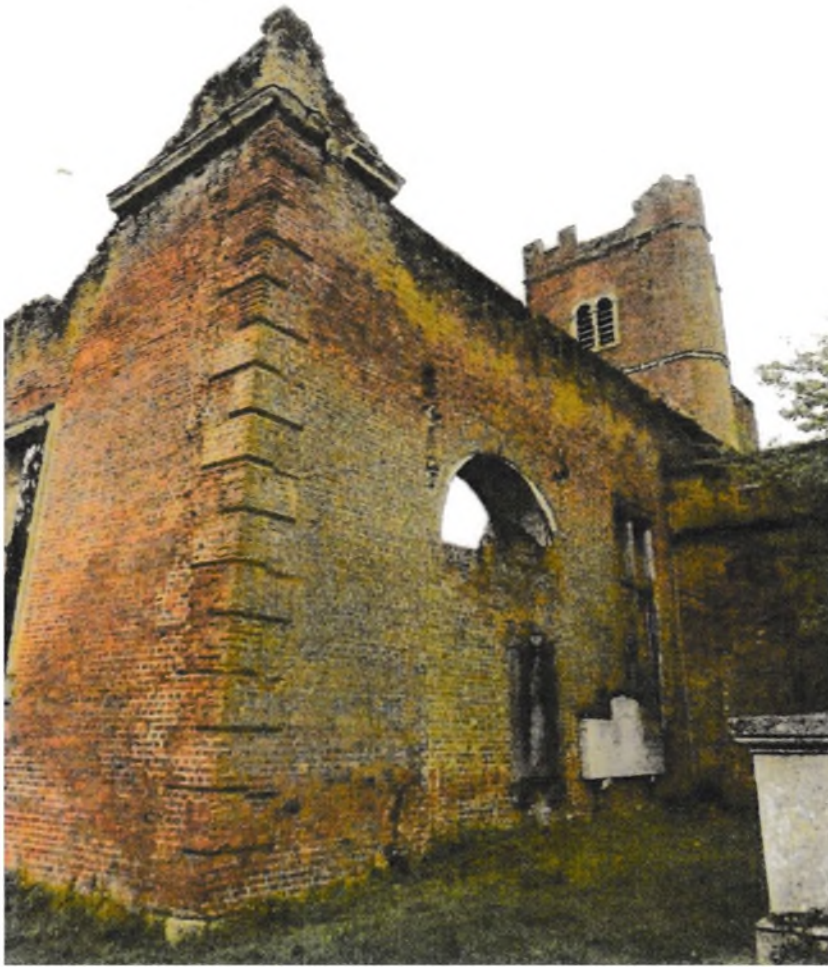
Fig.7 The rusticated north-east corner is sinking into the underlying soil. Four types of chamfered brick were made and these occur on all four external corners of the church. All photographs: Mike Chapman
