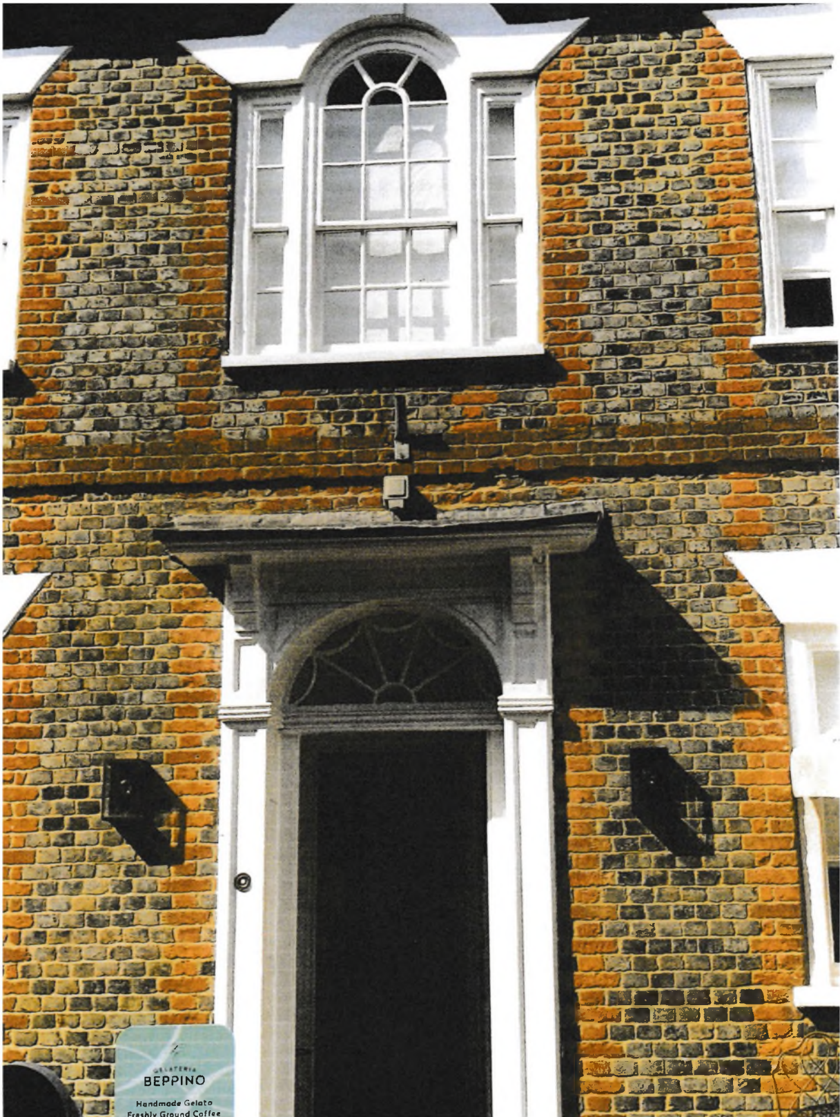
Fig.3 No. 33 West Street, Bridport, showing the overall extent in the centre of the façade of house of the use of blue brick in Header Bond with red brick used for window surrounds and the plat band.
