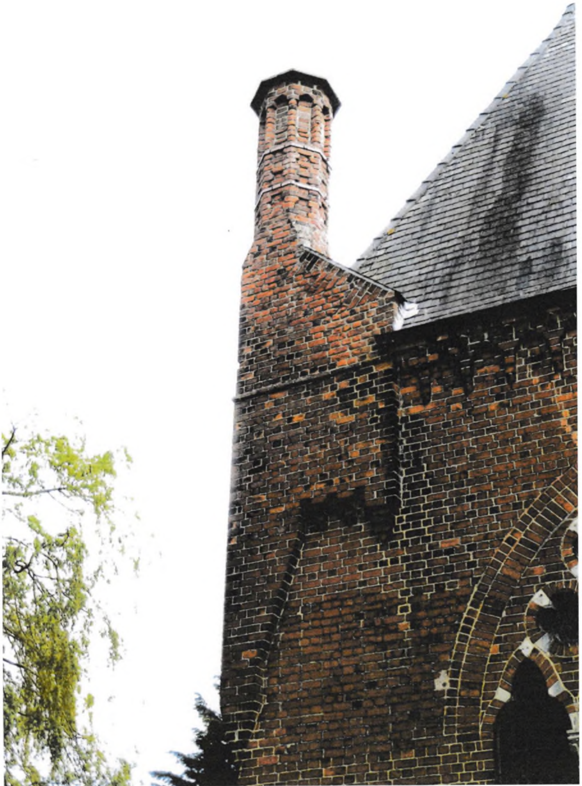
Fig.6 Burringham church: chimney at the north-west corner of the tower. The flat capstone replaces a cowl.
