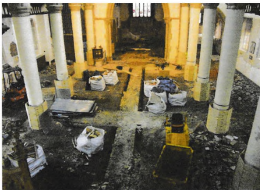
Fig.1 View of the floor of All Saints church, Wokingham, after the removal of wood blocks and tiles but before excavation.
