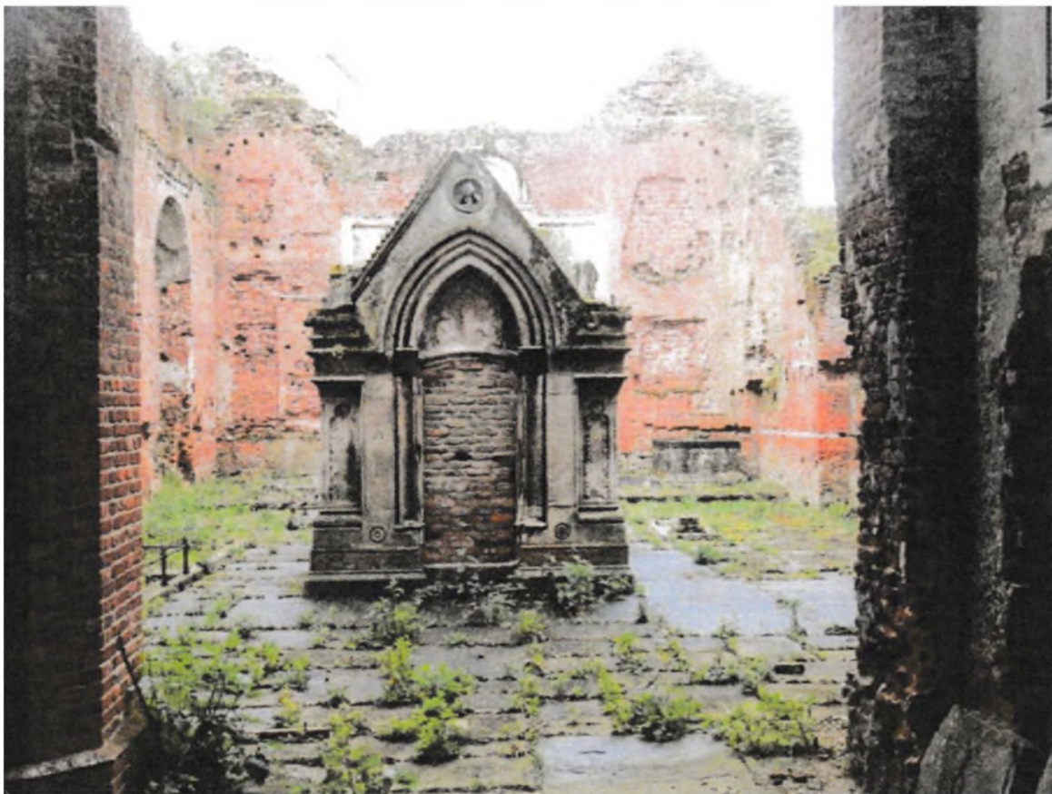
Fig.10 The Holland monument erected after the abandonment of the church in 1850. Note the scars on the east wall showing how earlier monuments were removed and transferred to the 1849 church adjacent.
