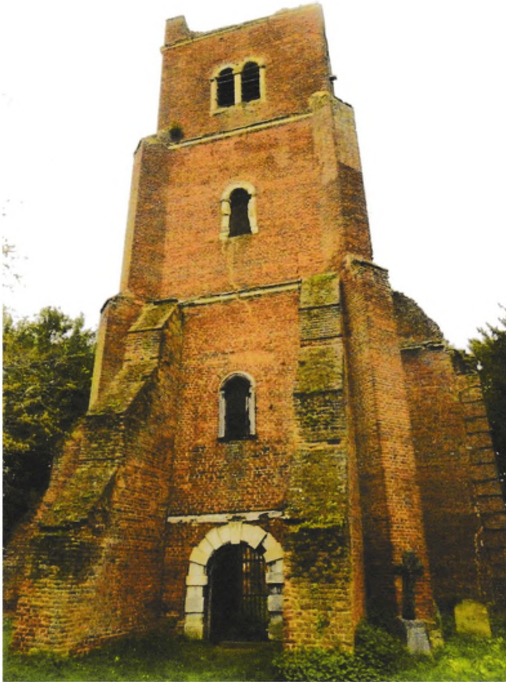
Fig.8 The west tower from the west. The diagonal buttresses at the corners are original; the two buttresses in alignment with the tower are eighteenth-century supports but not bonded into the original brickwork.
