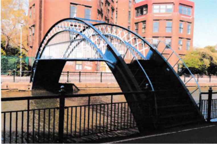
Fig.9 The Montague Street Bridge, Lincoln, with alternate steps by Fambrini & Daniels, erected in 1878.
