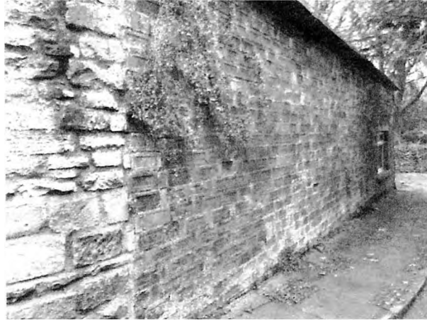
Fig.2 The brick wall at the entrance to the Greenfoot public car park in Settle, North Yorkshire. Photograph: Mike Chapman
