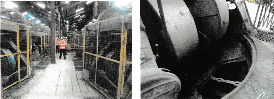
Fig. 9 (left) The “battery”of 16 Incla Dry Pans with the (right) A pan under maintenance, showing the all important pan floor,with two base sections removed.
