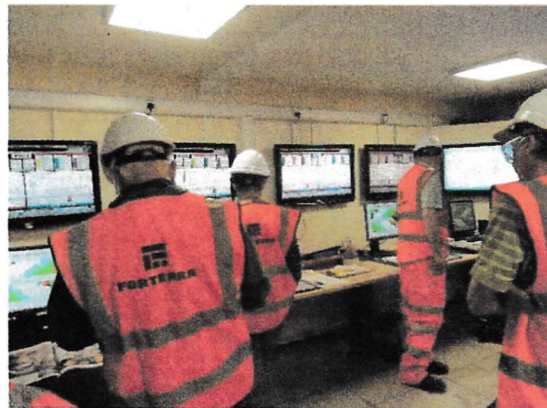
Fig. 19 The bank of computer screens displaying every stage of the firing process, giving continuous insight into what is happening at each stage of the firing process
