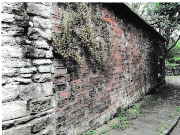
Fig.1 The brick wall at the entrance to the Greenfoot public car park in Settle, North Yorkshire.
